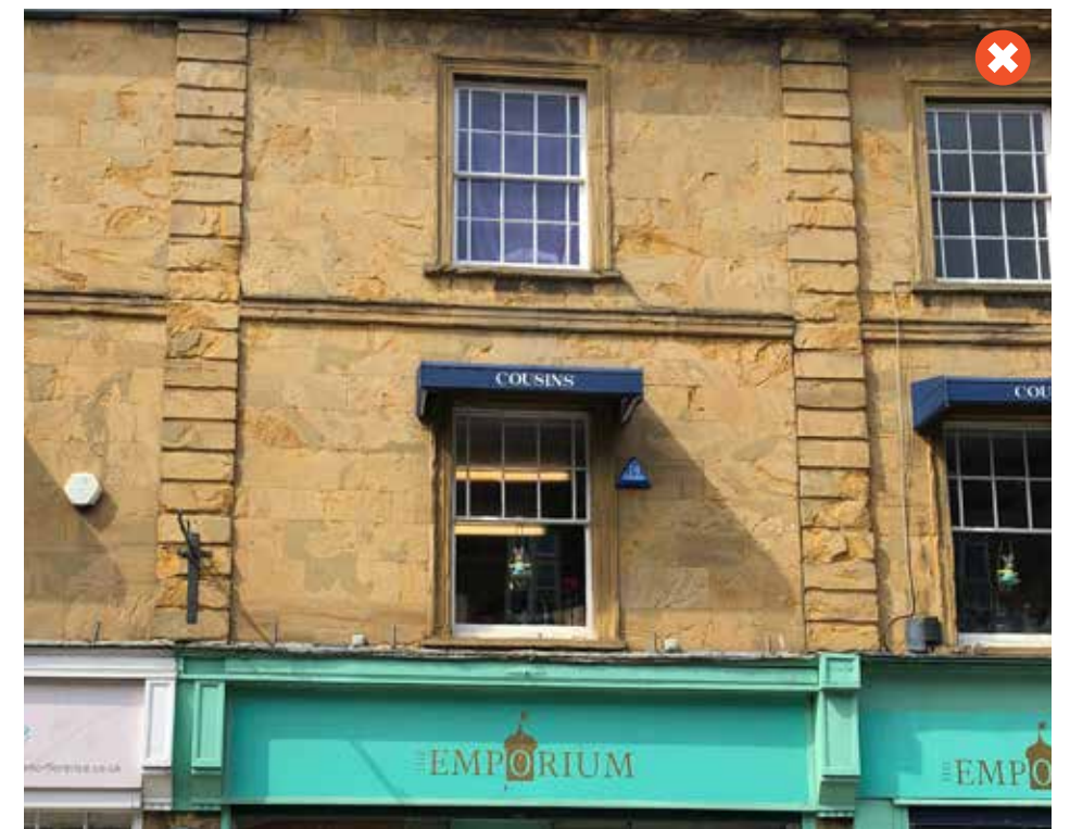
Figure 54. Alarm boxes haphazardly positioned on facade
