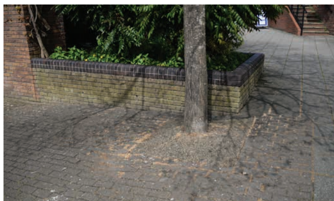
Existing tree roots damaging paving area
