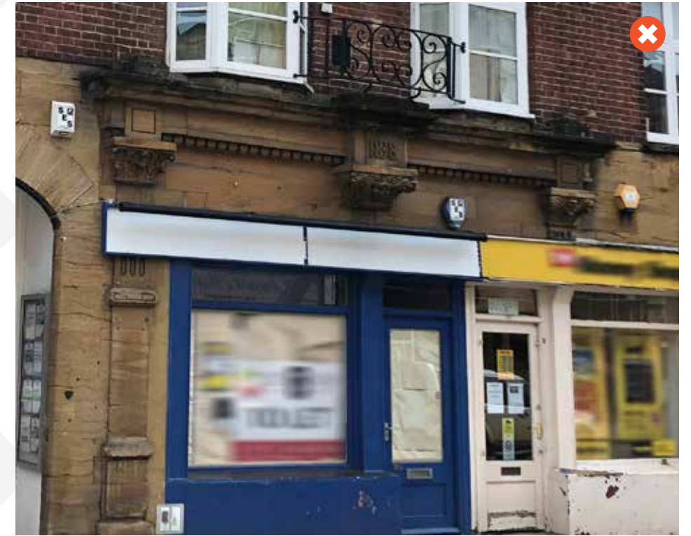
Figure 51. Alarm boxes haphazardly positioned on facade
